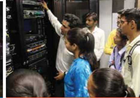
BSNL Ahmedabad Networking & Telecommunication server room
